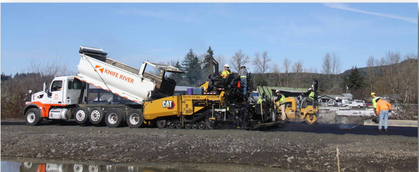
Knife River employees pour asphalt in February at the new Linn County Parks RV dump.
